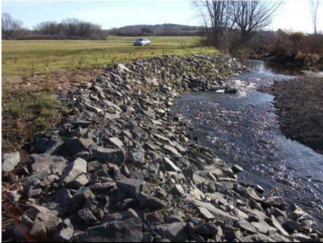
Picture 2: A stabilized bank at Lisson Dale Black Angus Farm that was stabilized. Small groynes further increase habitat and channel stability
